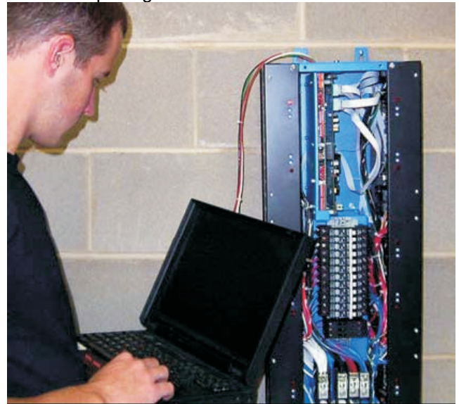
Uploading lighting changes to the dimming panel
